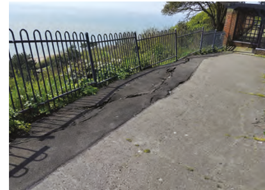
Slope failure on coastal footpath
