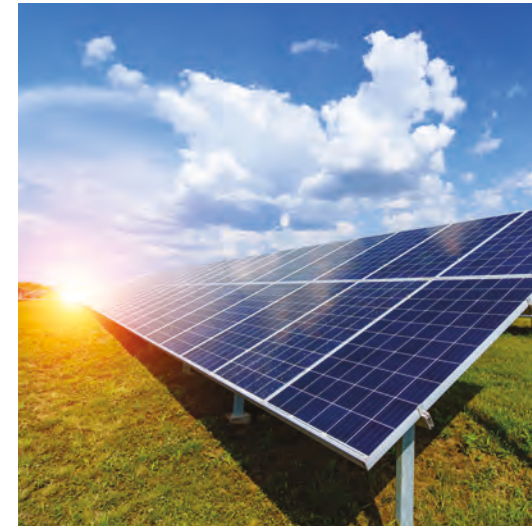
Solar PV farm
