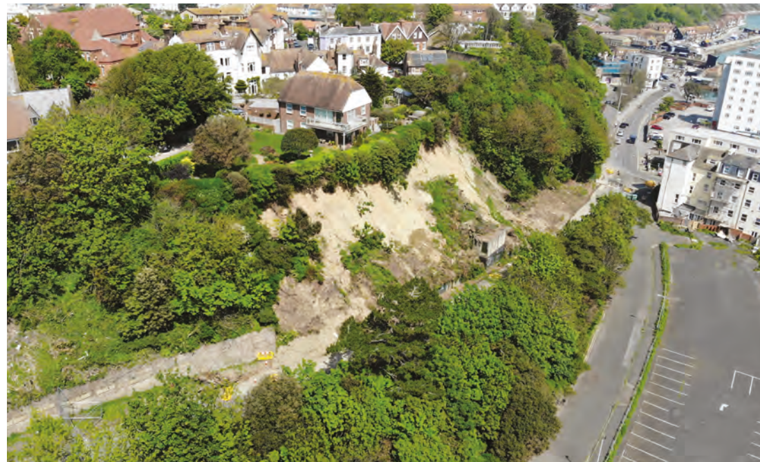
Slope failure adjacent to residential property
